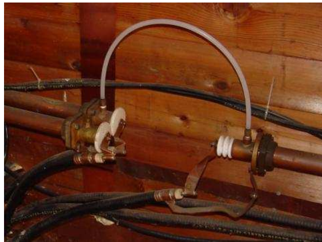
Figure 14.52: Flexible coaxial cables connected to rigid lines.
